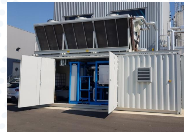
Heat recovery on Incinerator– 180kW ORC - France
